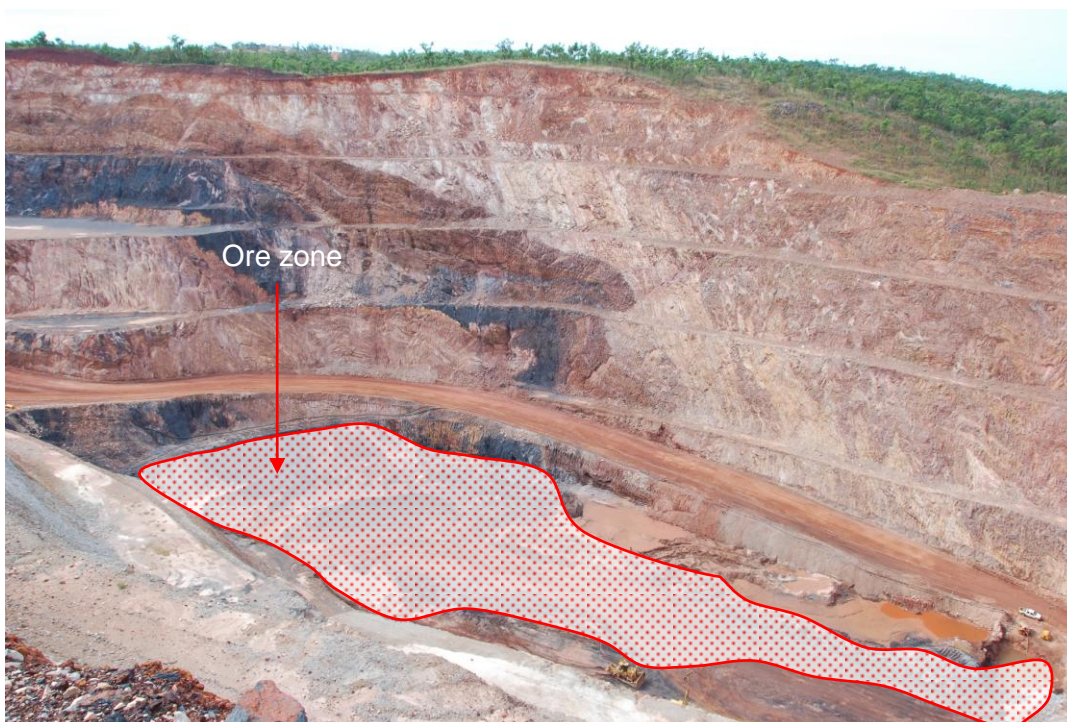
Figure 8 - Eastern Pit at the end of June 2010 looking north-west showing bench development
