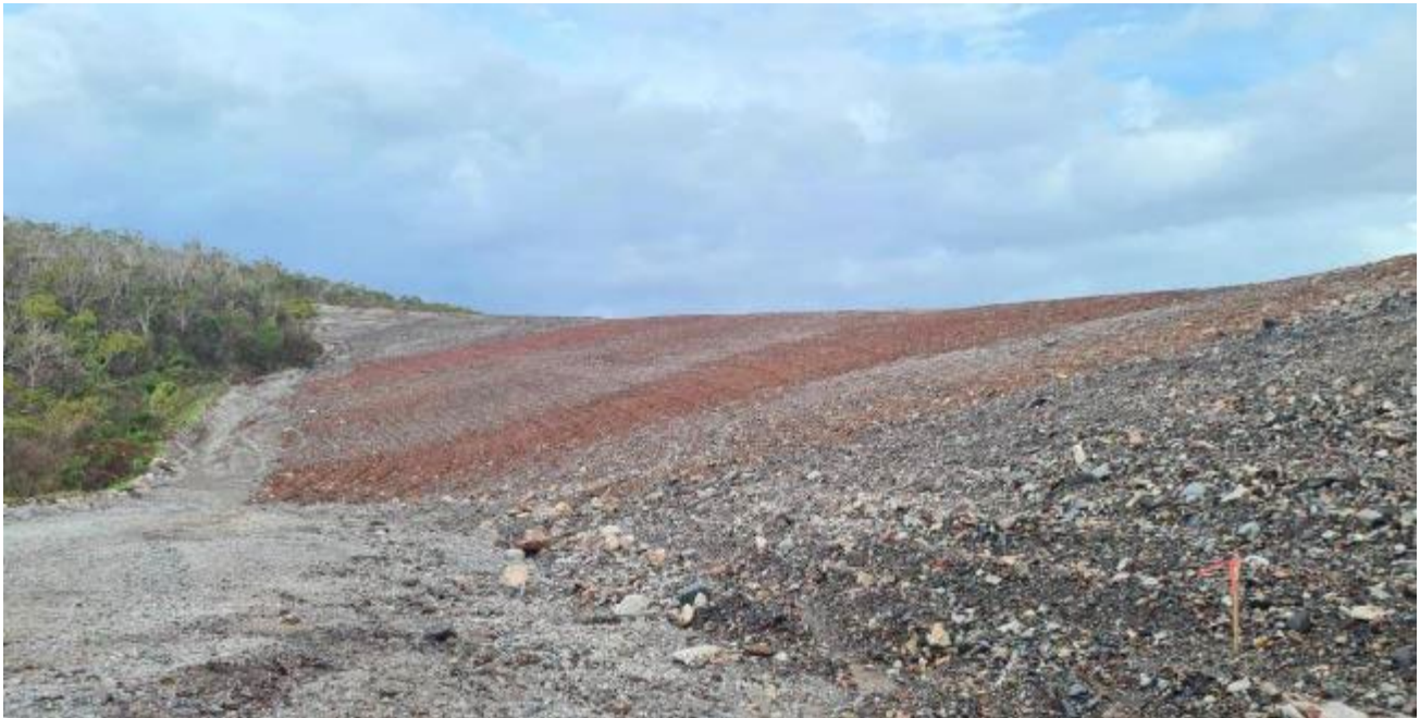
Figure 99: Slope post rainfall, Late February 2024.
