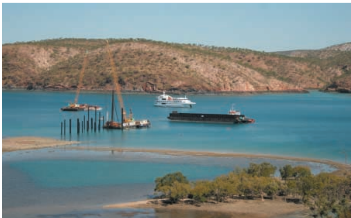
From Construction to Production: Almost 50% of the jetty piling is complete on Koolan Island.
